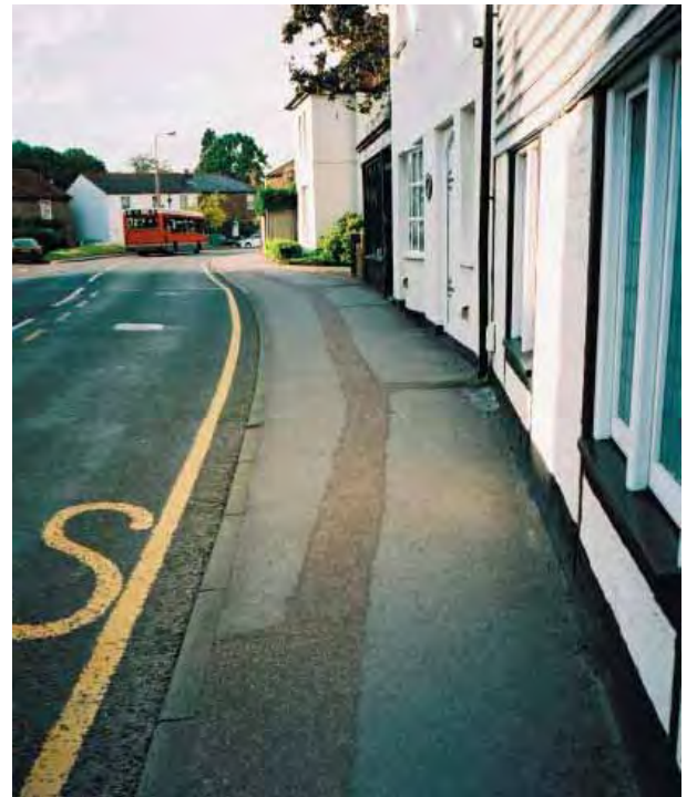
Poor quality paving in Bridge Road.
